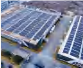
Rooftop PV System at Chuxiong Base
