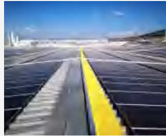
Rooftop PV System at Yuhuan Base
