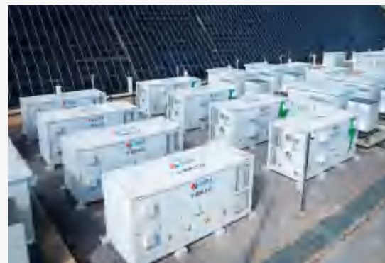
Xiaoheima "PV + ESS" Project
