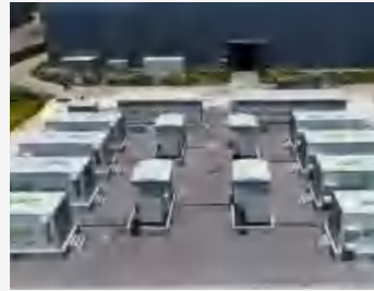
ESS Project at Haining Base
